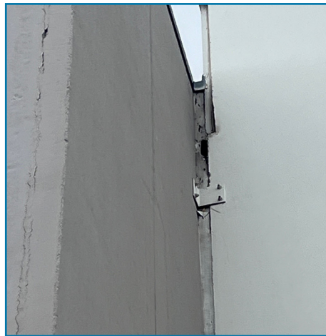
Structural Movement: Building panels can move in some cases. During our inspections we attempt to determine the cause, then present repair solutions.
