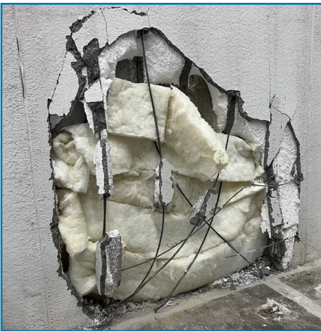
Impact Damage: Many times, buildings are damaged due to vehicles impact. Most of the time this type of damage is not structural and can be easily repaired.
