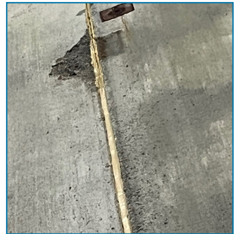
Interior caulk joint and cracked concrete: When panels move caulking joints and weld plates may fail. When this occurs the weld plates and caulking joints require repair.
