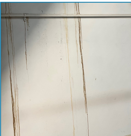
Staining: This indicates that water has leaked into the building. Water can cause damage to the panels and to other material on the inside of the building.
