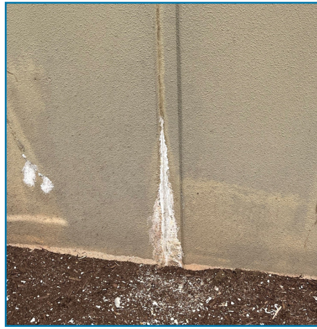
Efflorescence: When there is a high presence of moisture, crystallized residue can form on the outside of the buildings. Left unattended, this can cause deterioration of the concrete.
