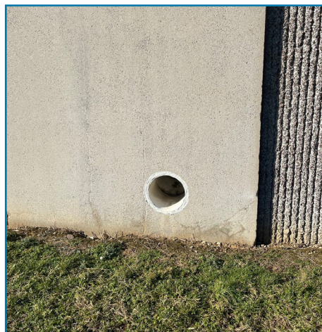
Poor drainage: Poor drainage leads to major issues such as cracked walls, failed caulking joints, mold, heaving concrete, and foundation problems.
