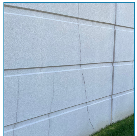
Cracks: Most cracks are superficial and will not cause structural problems. This is an inherent part of concrete construction. However, some cracks are much worse and require repair.
