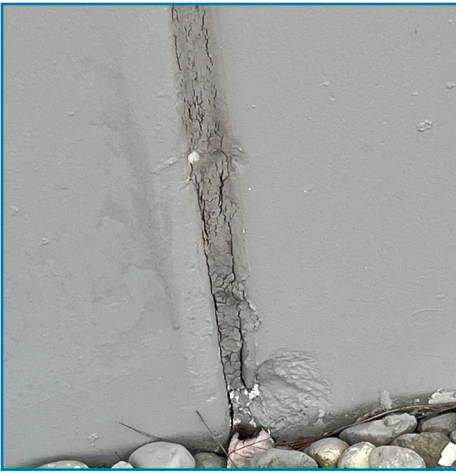
Caulking failure: This occurs when caulking has reached its lifespan, approximately 10 years. Left unattended moisture and air enter into a building causing additional damage.
